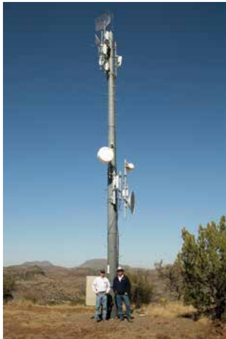
Tower with backhaul and Access Points
